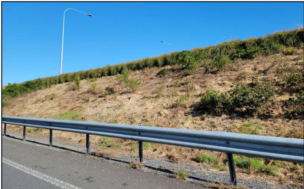
Figure 3: Landscape planting on Mackays to Pekapeka expressway where the mitigation planting has died and is now rank grass interspersed with the plants that have survived.
